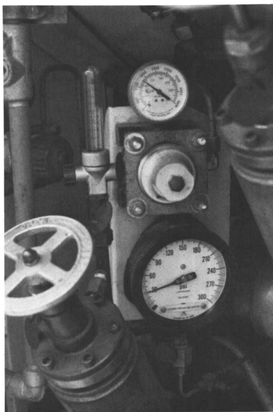
Figure 18. Helium purge controls
